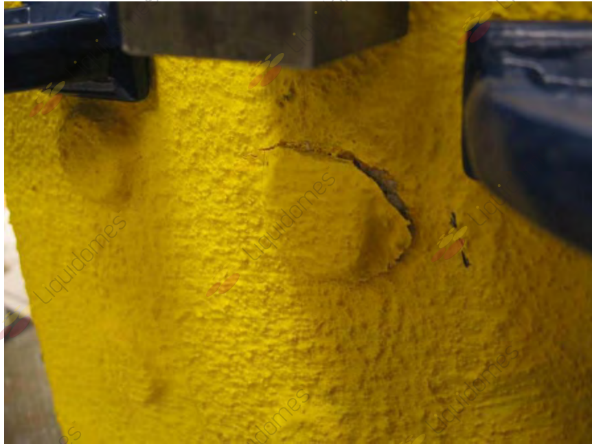
Photo No. 5 Bond Strength Failure Detail
